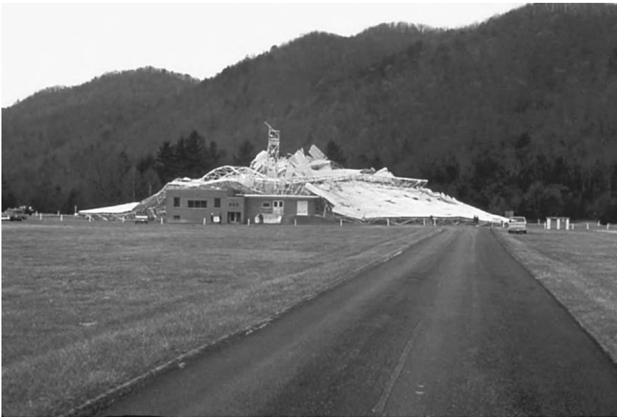
FIGURE 15.1. At 9:43 pm EST on Tuesday the 15th of November 1988, the 300-ft telescope in Green Bank collapsed. The collapse was due to the sudden failure of a key structural element—a large gusset plate in the box girder assembly that formed the main support for the antenna. This is a photograph of the 300-ft telescope taken on November 16, 1988 after the collapse. The loss of the 300-ft telescope resulted in the Green Bank Telescope project, Figure 15.2. (Photo Richard Porcas, courtesy of the NRAO/AUI.)
