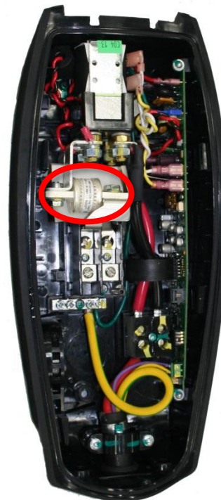
Figure 2 (HPWC with 200A fuses)
