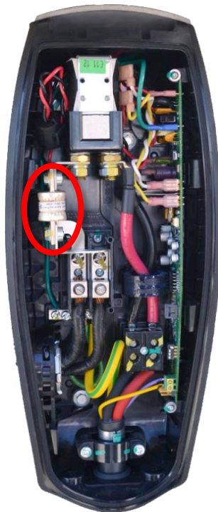
Figure 1 (HPWC with 100A fuses)
