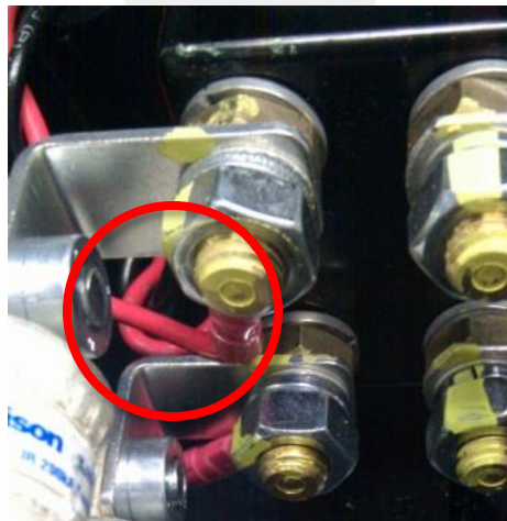
✘ Figure 19 (Incorrect: resting on bus bar)
