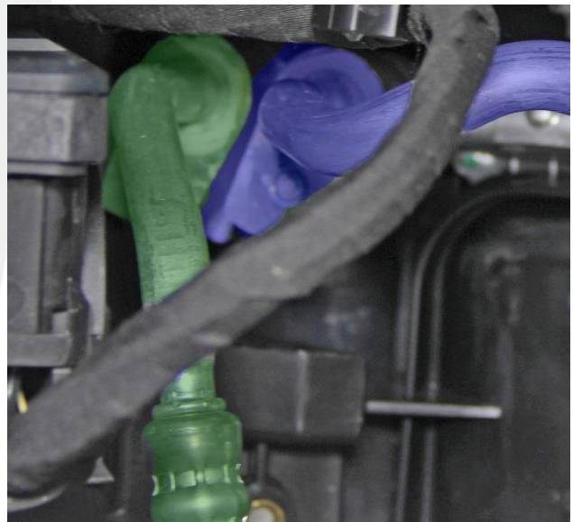
✗ Figure 3 (A/C condenser pipes highlighted)
