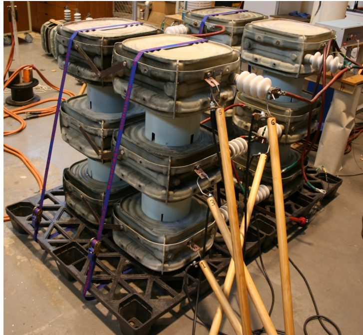
Figure 3.7 The prototype 90 kV capacitor bank, using PVC pipe insulators. Six earth sticks are applied to the bank to individually short out the capacitors.
