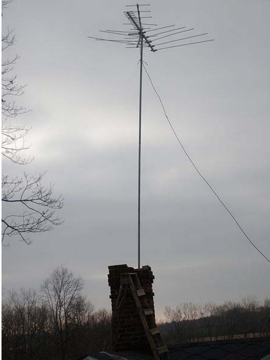
An antenna pole setup in a chimney, reaching 35 feet (10.7 meters) off the ground
