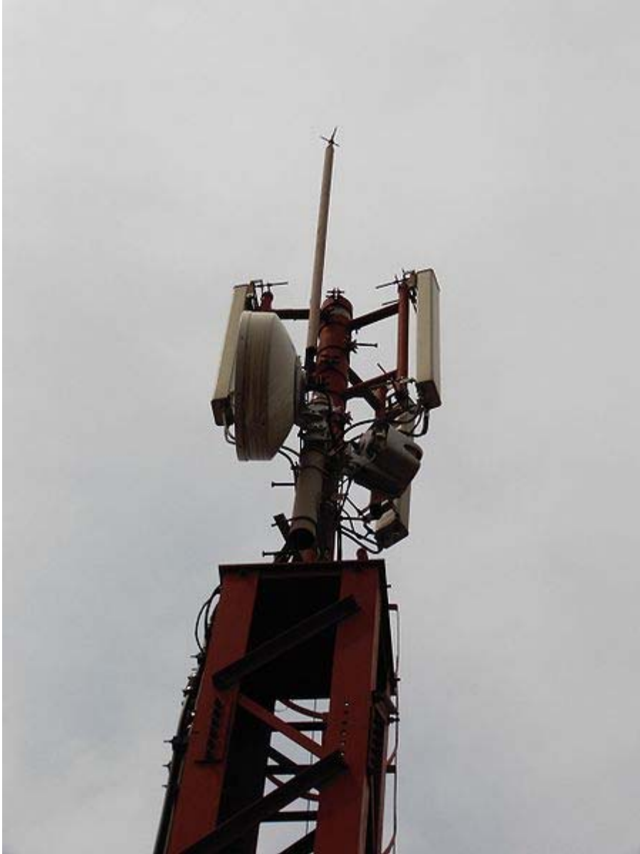
A three-sector telephone site in Mexico City.
