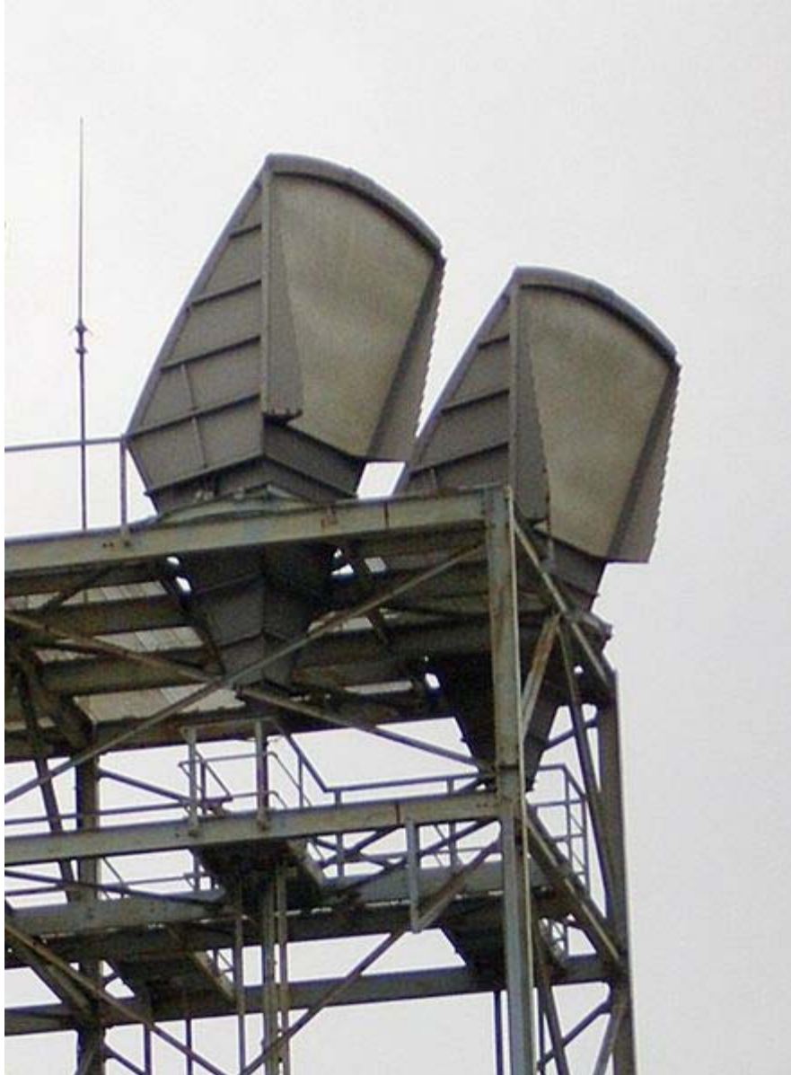
Hogg microwave relay antennas on roof of AT&T telephone switching center, Seattle, Washington, USA Hogg antennas
