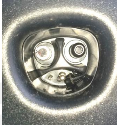
Figure 5 (Dislodged pin deadfront at lower right)
