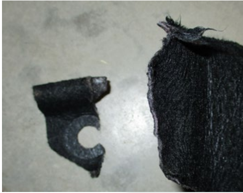
Figure 4 – Panel Tearing at Fasteners; Replace Panels
