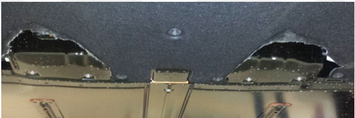
Figure 6 – Panel Separation At Leading Edge; Replace Panels
