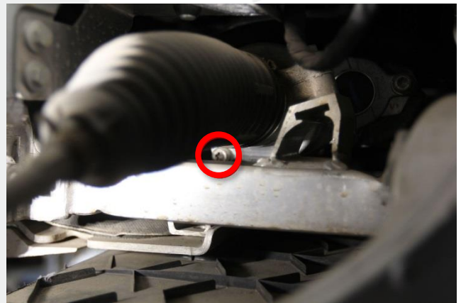
Figure 2 – Steering rack housing bolt 4
