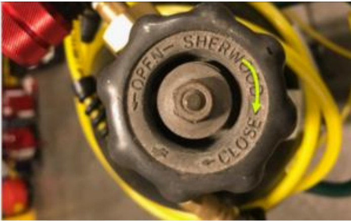
Figure 7 – Main Supply Valve
