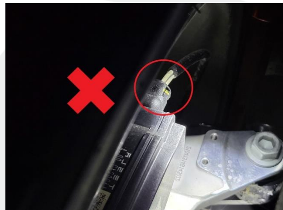
Figure 3 – Corrugated tubing not installed
