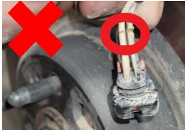
Figure 4 – EPB wire insulation damaged
