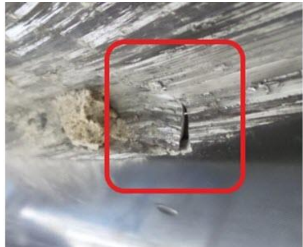
Figure 2 – Visible open crack
