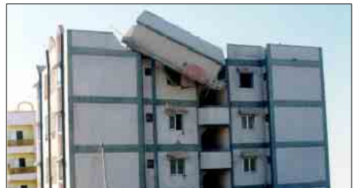
Fig 4.16: No Support for rooftop water tanks
