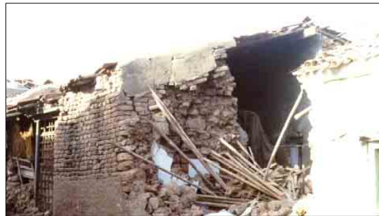
Fig 4.7: Collapsed Unreinforced brick house
