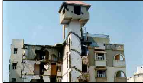
Fig 4.15: Inadequate transfer mechanism
