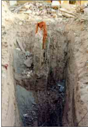
Fig 4.13: Absence of plinth beams
