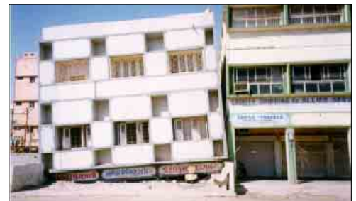
Fig 4.17: Collapsed soft stories
