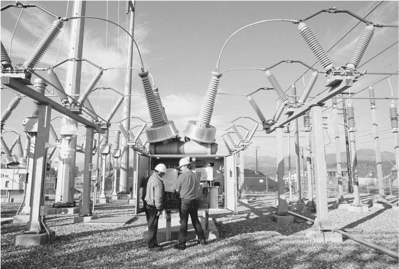
Pend Oreille Utility District workers at a control box in a power substation. (Corbis-Bettmann)
