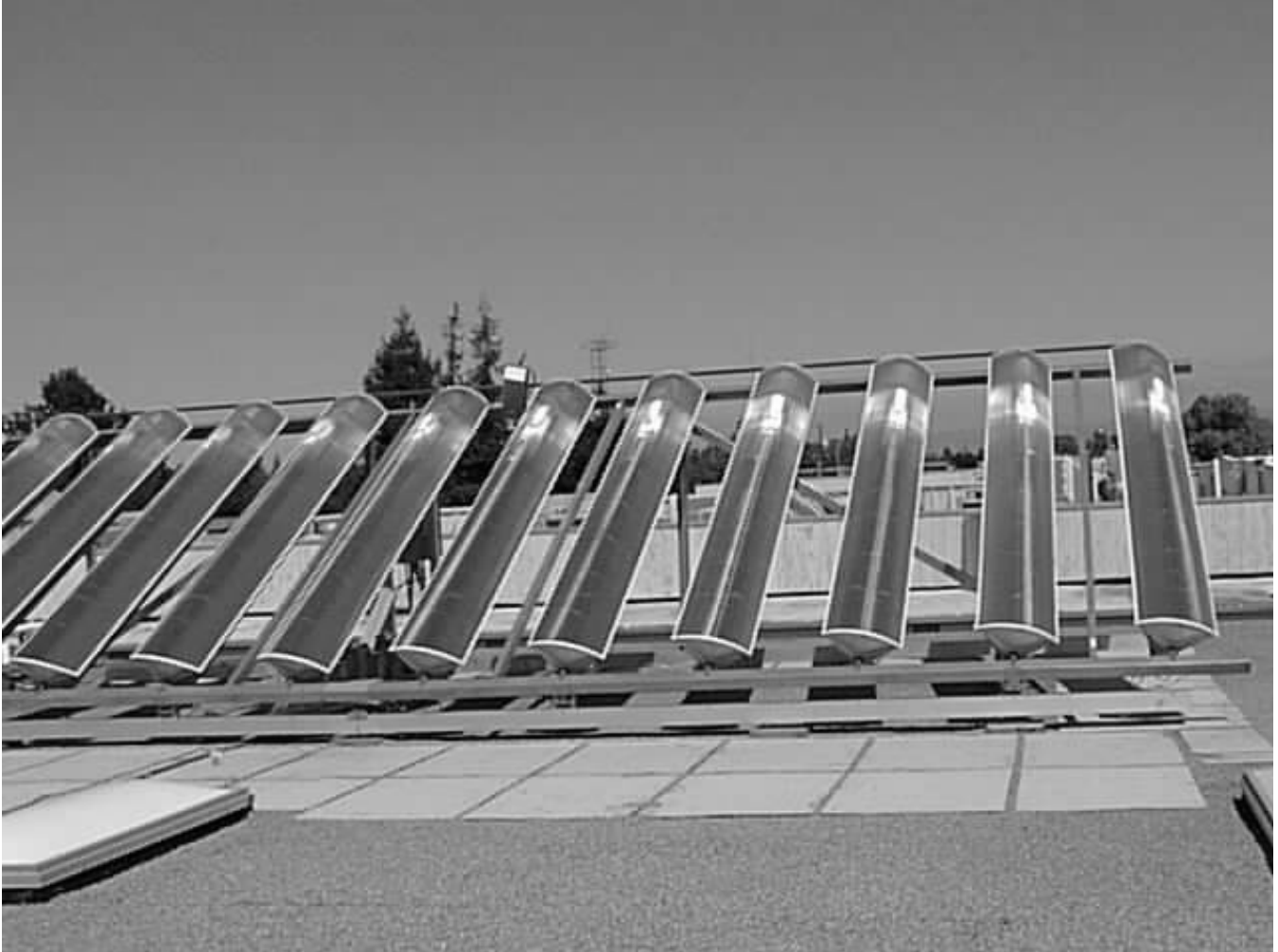
Figure 3, Powergrid Panel on the Roof of the PVI Building
