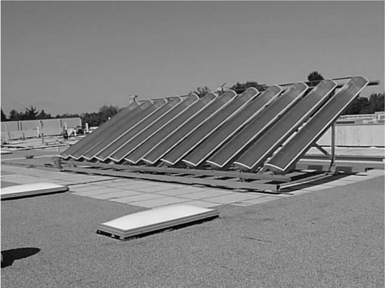
Figure 1, New PVI Powergrid on PVI Roof
