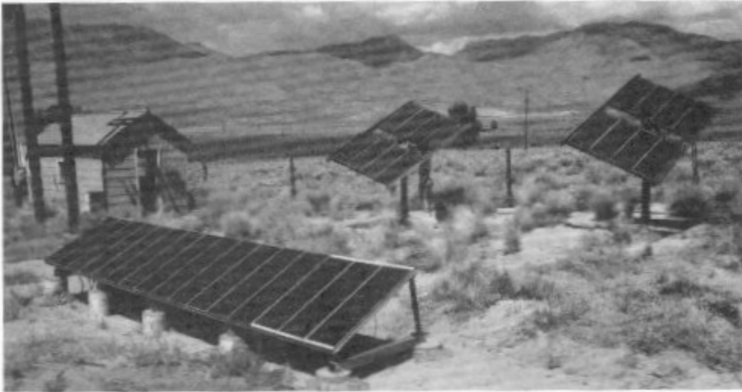
FIGURE 11.24 Two types of solar photovoltaic collectors at a remote site in Bishop, Calif. (Courtesy of Southern California Edison.)
