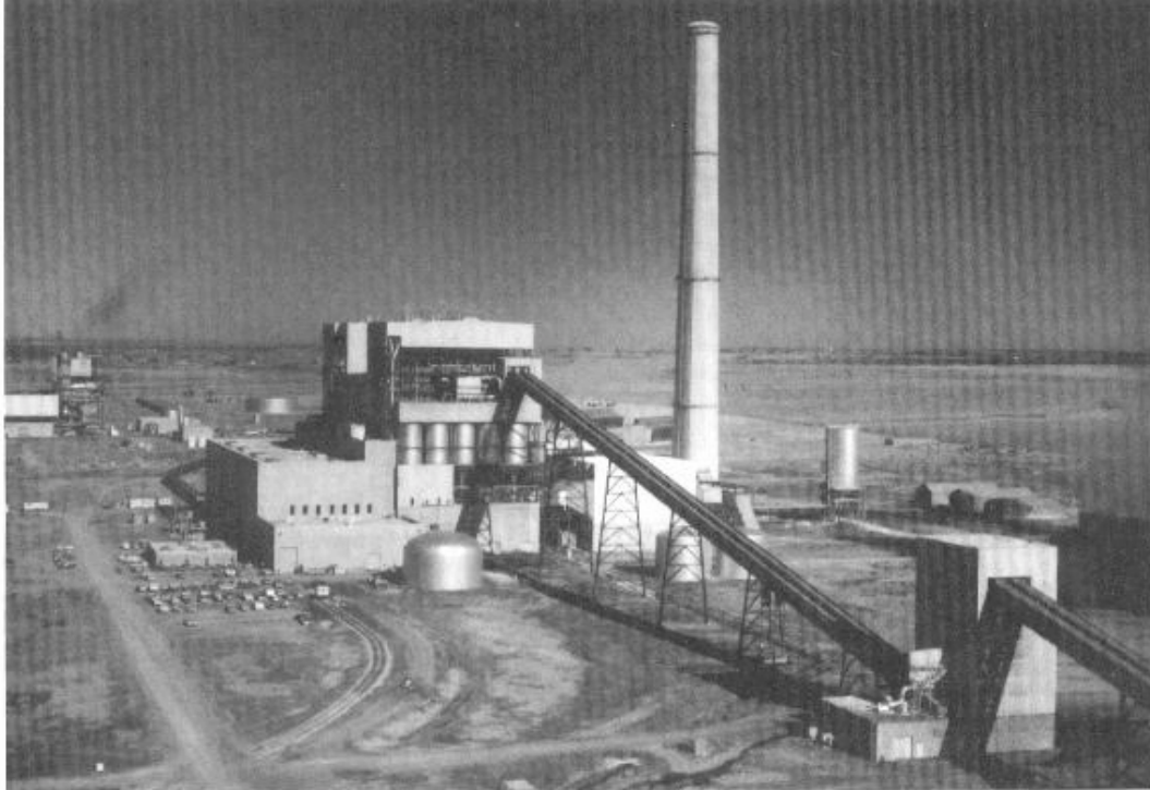
FIGURE 2.1 A modern coal-burning steam power plant nearing completion. Coal is transported by conveyor from the storage pile to the crusher building at lower right, to silos visible on the side of the steam generator at the far end of the conveyor. The turbine room is to the left of the steam generator. Cooling towers at the extreme right cool the condenser cooling water. A 1970-vintage natural-gas-burning plant is visible in the left rear. (Courtesy of the Public Service Company of Oklahoma.)
