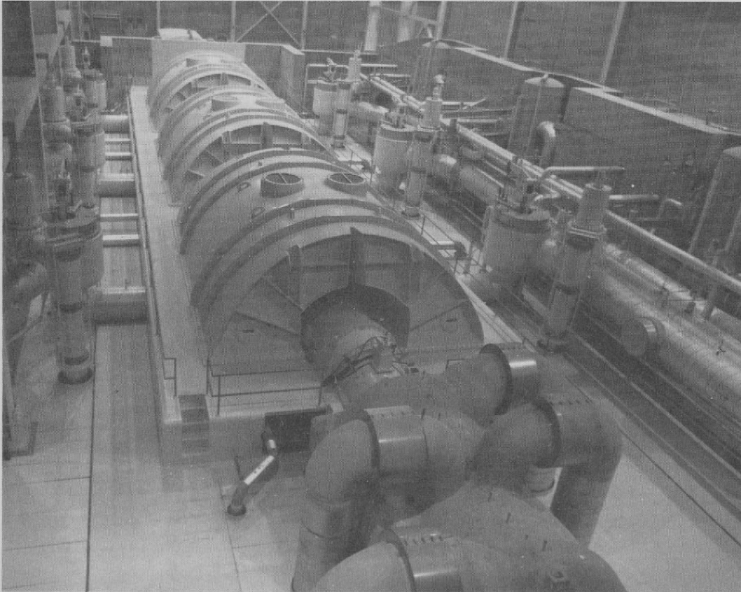
FIGURE 4.7 Turbine room at TVA's Brown's Ferry nuclear power station. One of the three generators can produce enough electricity to satisfy the residential needs of a small city. (Courtesy of the Tennessee Valley Authority.)
