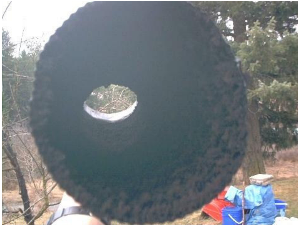
This chimney pipe is restricted by creosote. This is a dangerous situation. The creosote restricts air flow and can ignite causing a disastrous fire.
