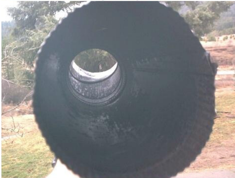
The same pipe cleaned of creosote. The air flow is much more efficient and no combustibles are present.
