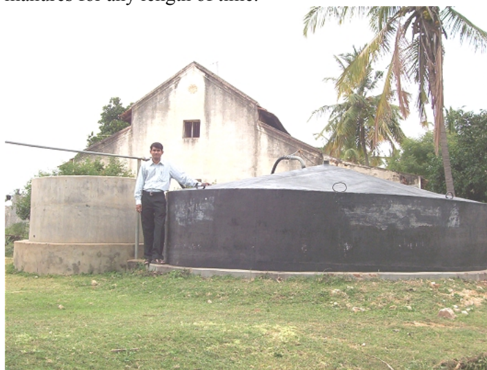
A continuous biogas plant
