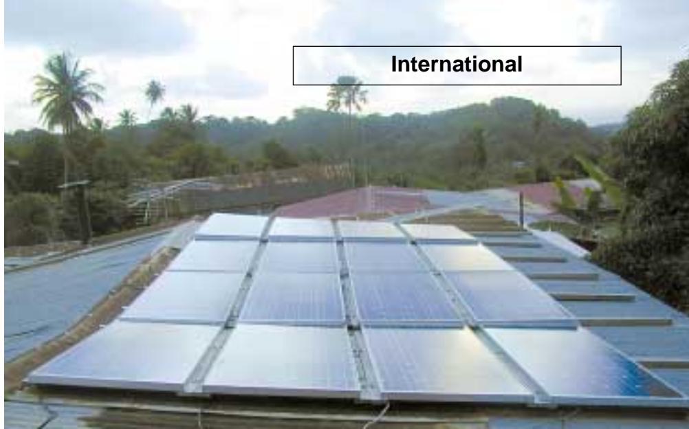
Sixteen, 120 watt AstroPower modules provide power directly to DC-driven, chocolate making machines.
