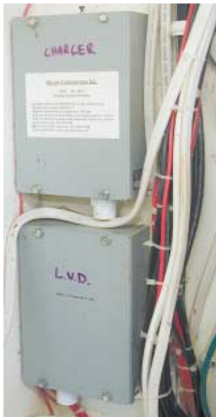
The voltage sensors and controls for the low voltage disconnect and AC battery charger.
