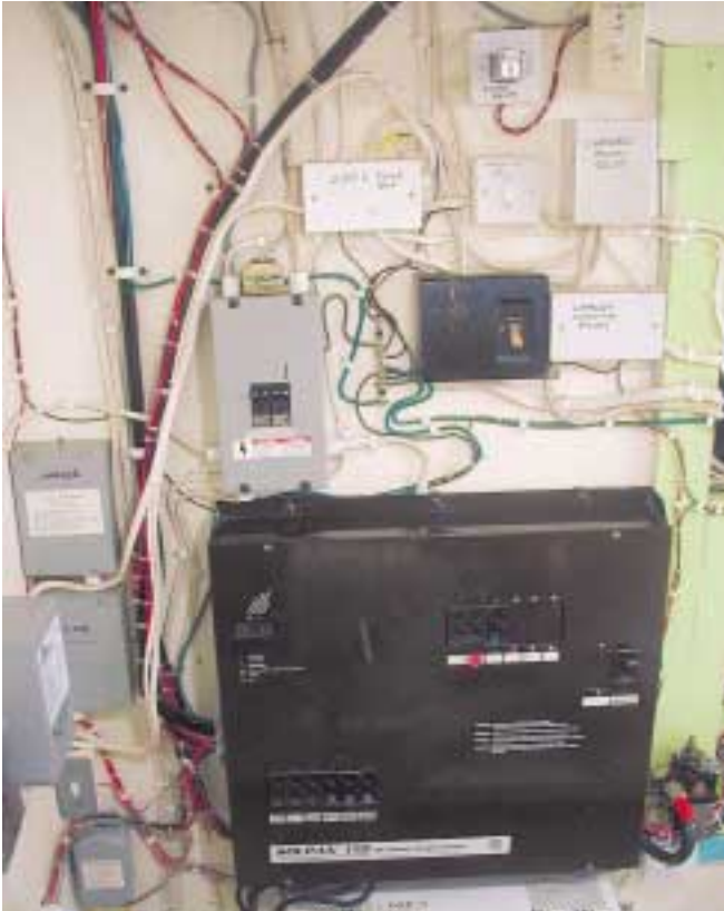
The power wall including the SolPan 110 DC load center, which contains a Heliotrope CC-120 charge controller.
