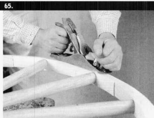
A smoothing plane is used to clean up the cut made by the power plane.
