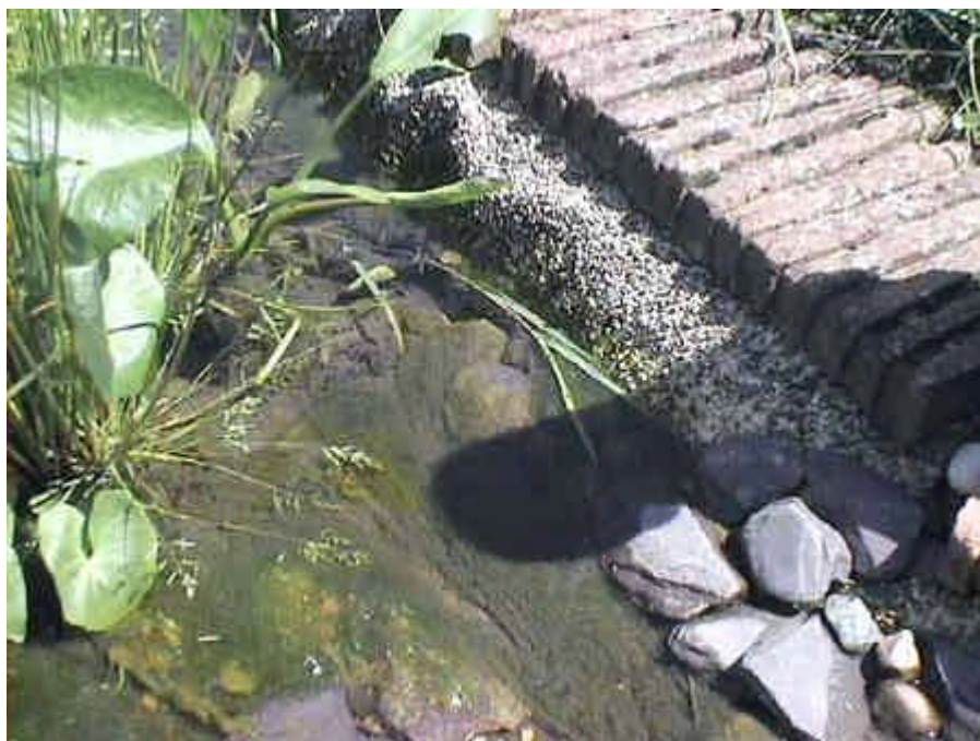
Close-up of the sides where the black liner is covered by the (expensive) gravel coated plastic.
