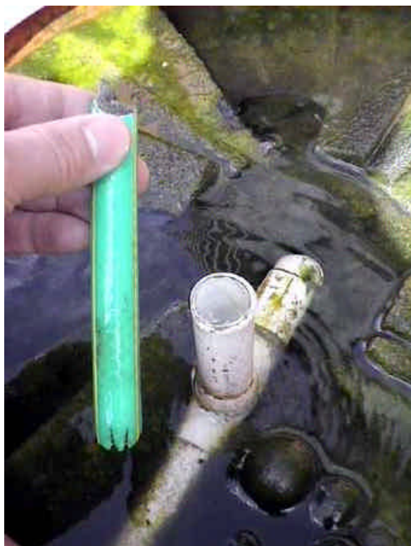
The length of hosepipe fits snugly into the 22mm standard plumbing pipe. I have not glued it because it means its dead easy to remove the venturi to clean the teeth each day, although often it works for 3 or 4 days without any attention.
