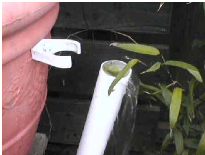
First I unclip the pipe, water starts to overflow.
