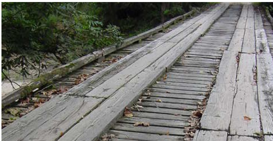
Wooden bridges are the easiest type to destroy; all you need is fire.
