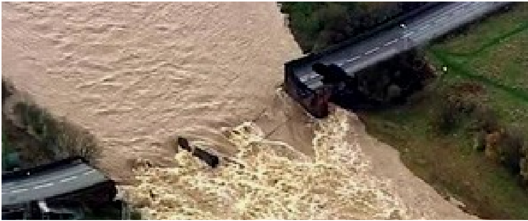
Bridge out, plus deep river, equals good roadblock.
