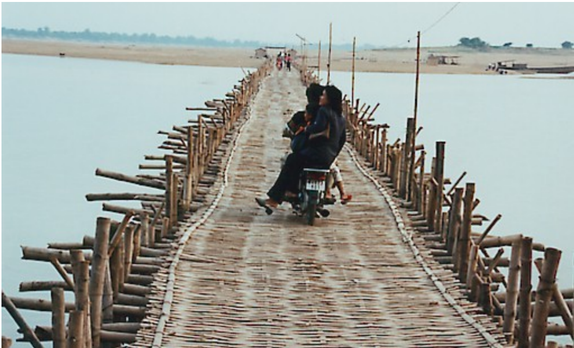
This bamboo bridge runs from the mainland to an Island, where the locals grow produce. Believe it or not, the bridge, which can support heavy cars and trucks, is dismantled every rainy season, to keep it from being washed away.
